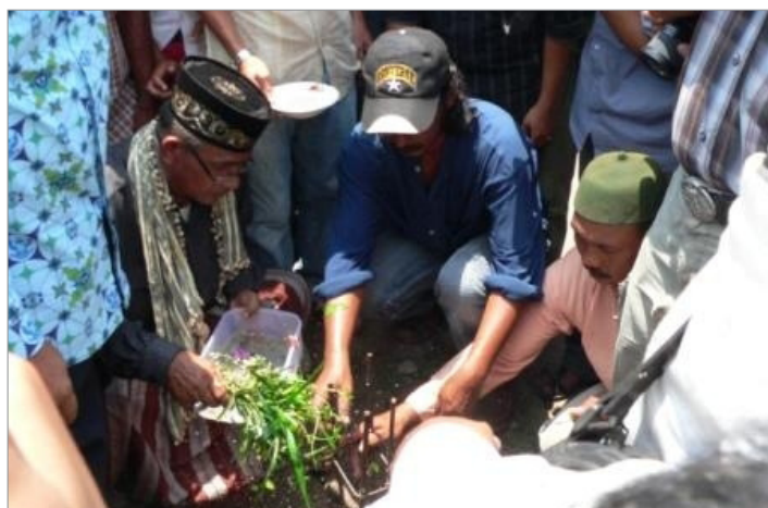
Local officials lay the foundation for a monument dedicated to the victims of the KKA Junction massacre.
